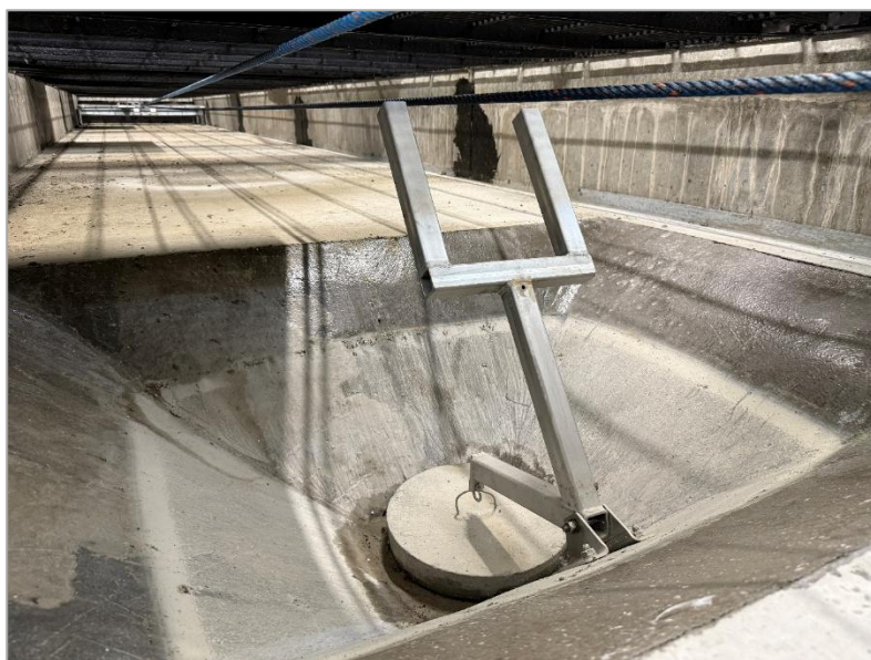
Figure 6 Automatic slurry discharge system, source: LJM Lind Jensen Agri.
