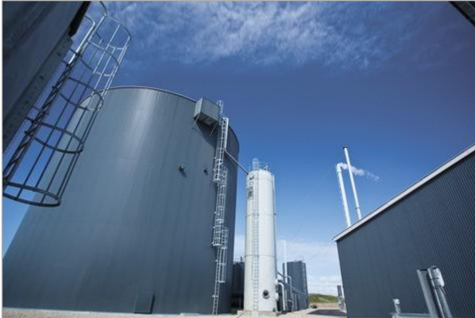
Figure 8 Biogas plant. Source: FBCD
