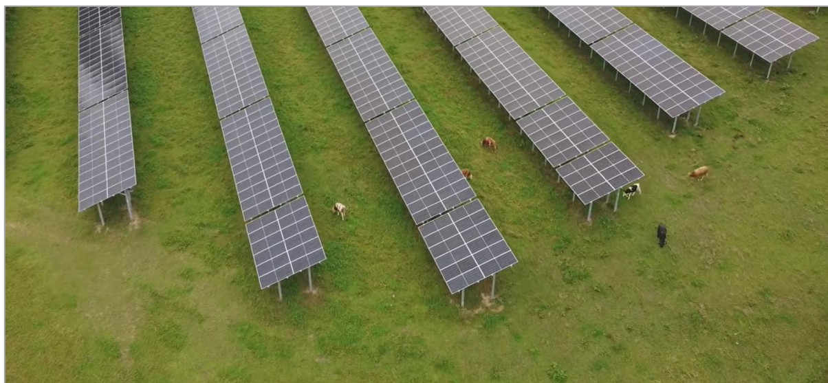
Figure 15 Agriphotovoltaic on a farm in Bavaria, Source: Regina Springer
